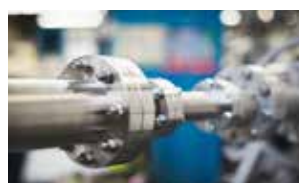
Processing Piping and Valves
